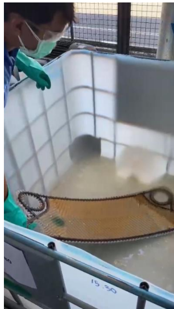
Gambar 3. Proses Perendaman Plat And Gasket Heat Exchanger
