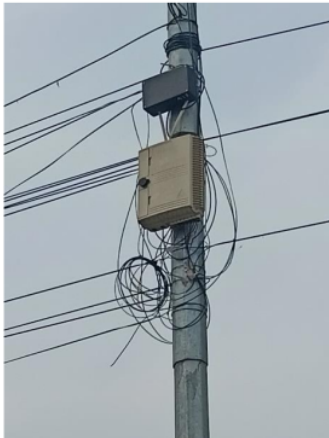
Router box wifi
